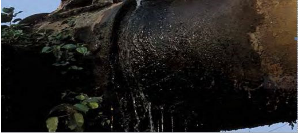
Fig. 11: Leaking water pipe (IRIN)
