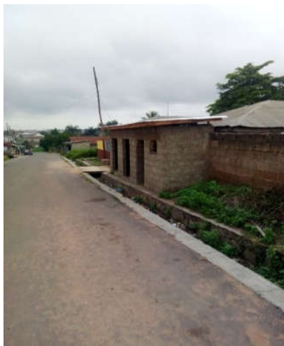
Plate 1: on-going construction of a shop building along Atukale Street off Yidi road Source: Fieldwork, 2019
